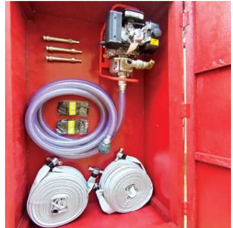
Fire-fighting equipment (Hariyama Plantation)
