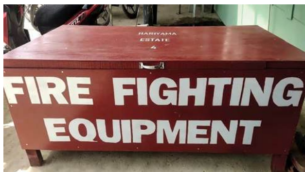
Fire-fighting equipment (Hariyama Plantation)
