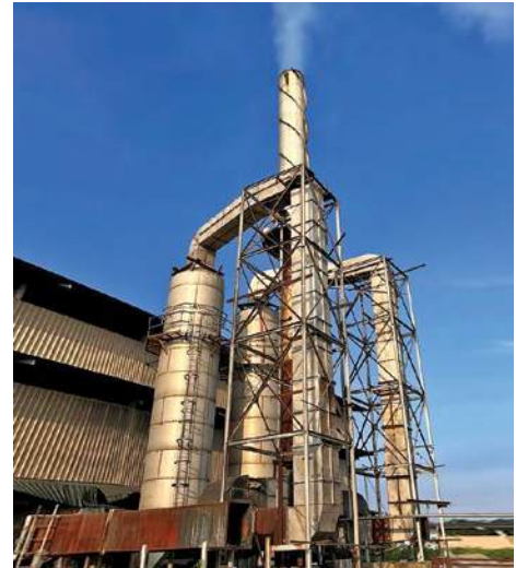
Scrubber system (Hariyama CPO Mill)
