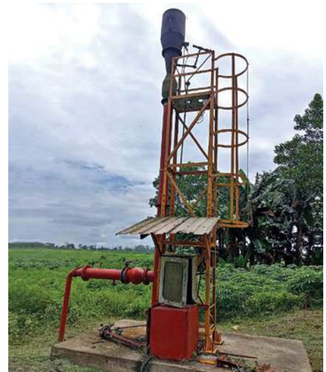
Biogas Flare Stack (Maujaya CPO Mill)
