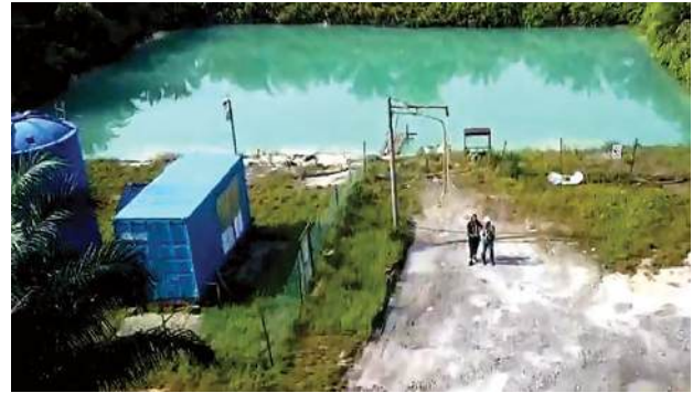
Water Treatment Plant (Sawai Plantation)
