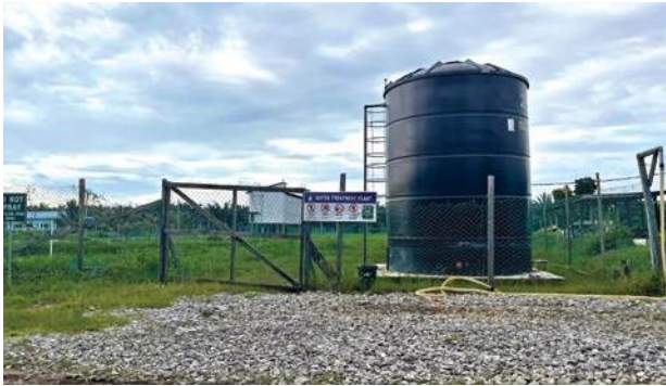
Water Treatment Plant (Poh Zhen Plantation)
